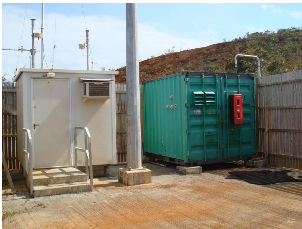
Figure 3: Station Prony Village
